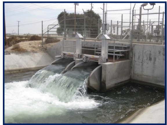
Figure 3-6. Flume Gates at Lateral Heading
