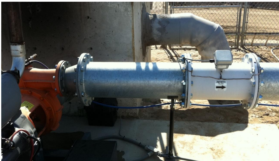
Figure A-6. Magnetic flow meter on delivery at Ra81.
