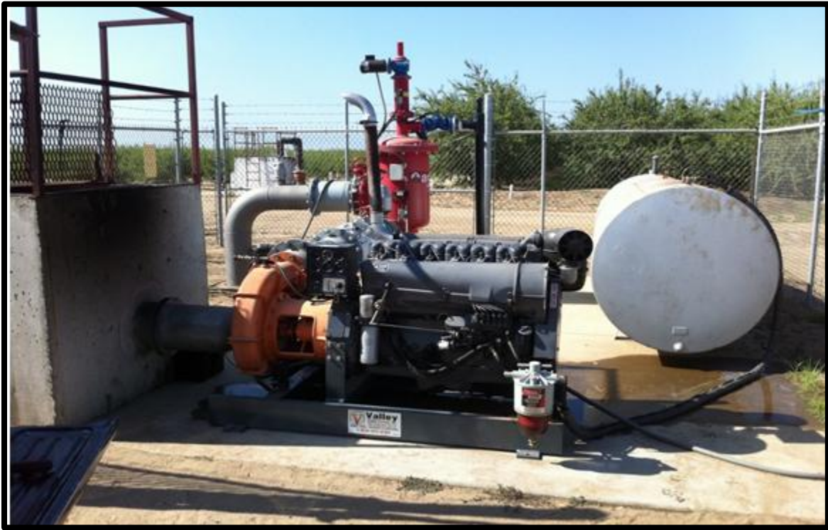
Figure A-2. Pump turnout on a District pipeline.
