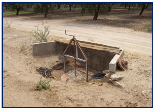
Figure 3-17. Orchard Valve Installed on SSJID Pipeline
