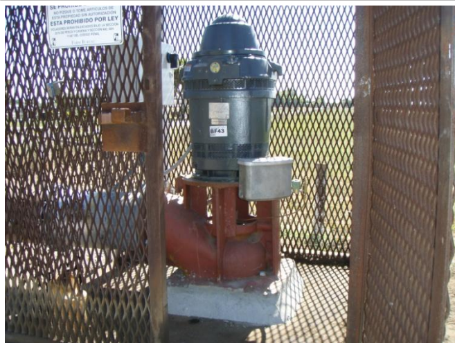
Figure 4-4. SSJID Groundwater Well
