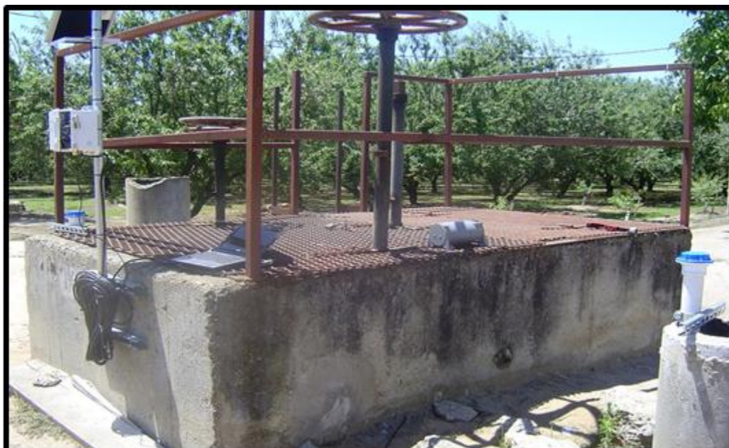
Figure A-4. Orifice gate turnout in a concrete box on a District pipeline.
