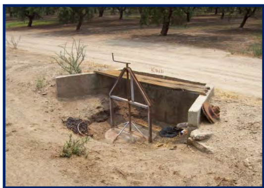
Figure 3-17. Orchard Valve Installed on SSJID Pipeline
