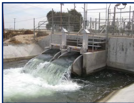
Figure 3-6. Flume Gates at Lateral Heading
