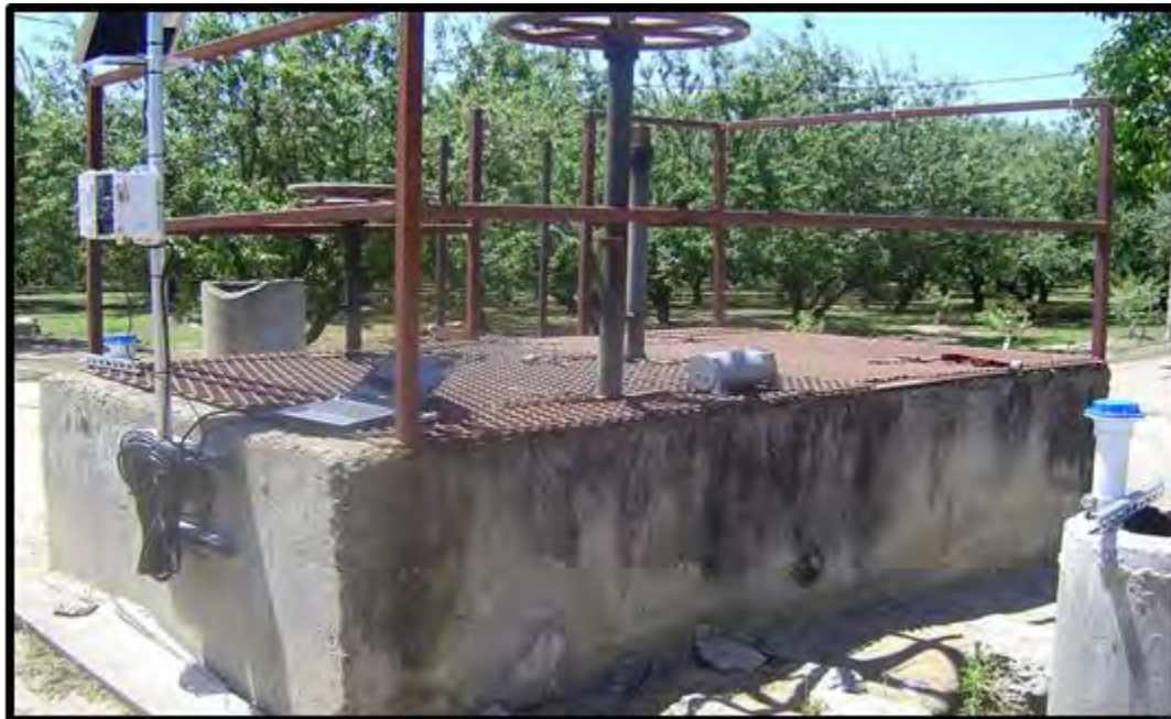
Figure A-4. Orifice gate turnout in a concrete box on a District pipeline.
