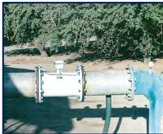
Figure 3-16. Magnetic Flow Meter
